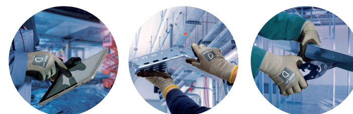
Work on display screen on site Cable path handling Partition wall assembly
